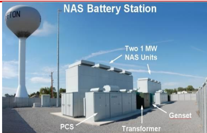
Three 2MW NaS Battery installations in AEP distribution system, 2008
